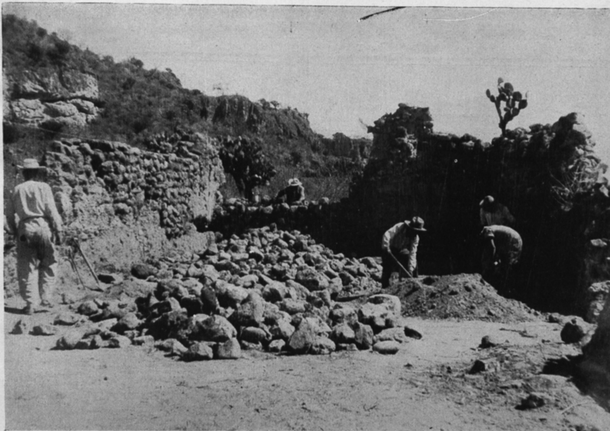
RECONSTRUCTION OF THE PALACE wall at Yagul, Oaxaca, is being done under the direction of Dr. Ignacio Bernal, head of the MCC anthropology department and director of Monumentos Prehispánicos. This building, which is the largest at the Yagul site, is exactly the same size as the famous Hall of Columns at Mitla. James Hester Photo
