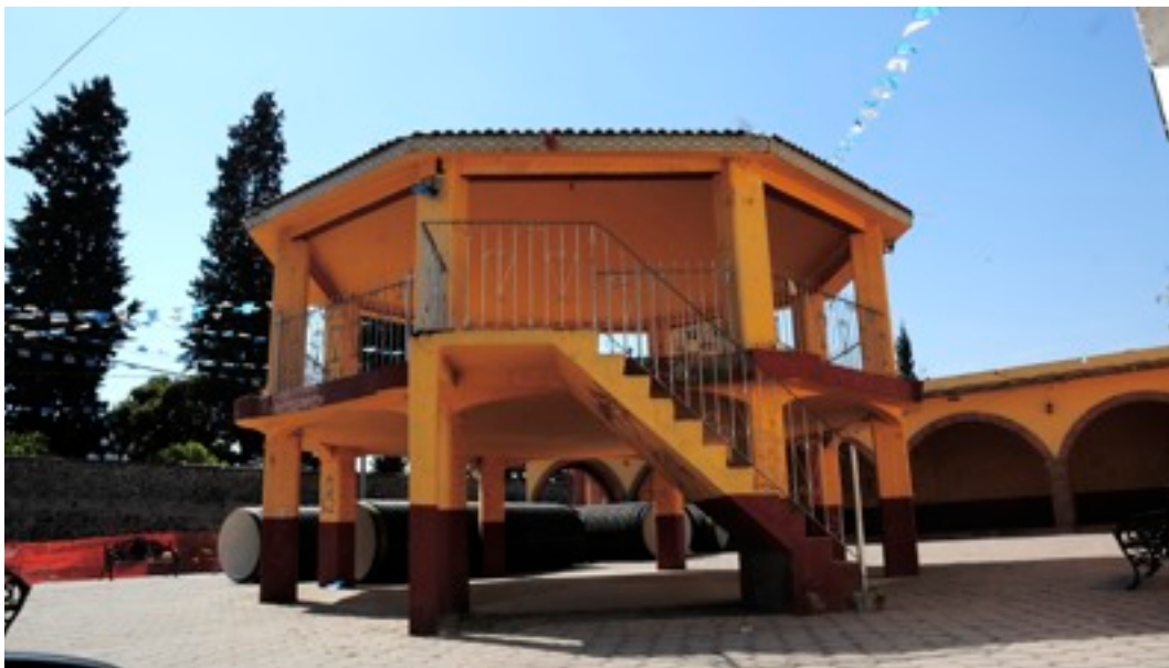
Santiago Xicotenco Kiosk. Deteriorated public space. San Andrés Cholula, Mexico. (Picture by Ramírez, 2013)
